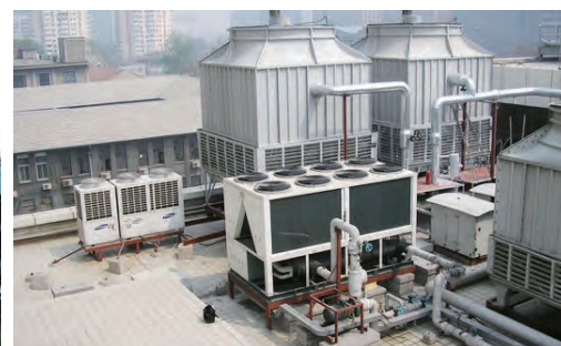
Noise Control of Commercial Building Equipment
