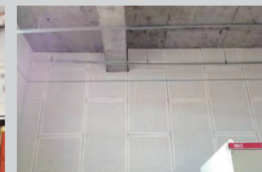
Indoor equipment room,workshop Computer room acoustic wall filled with sound-absorbing material
