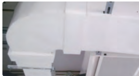
External protection of air duct system
