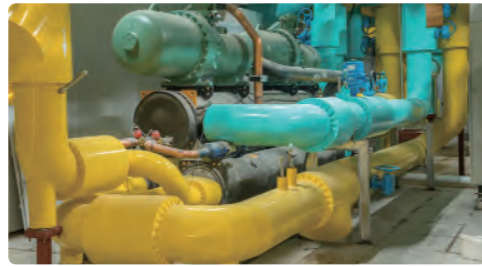
Irregular pipe external protection
